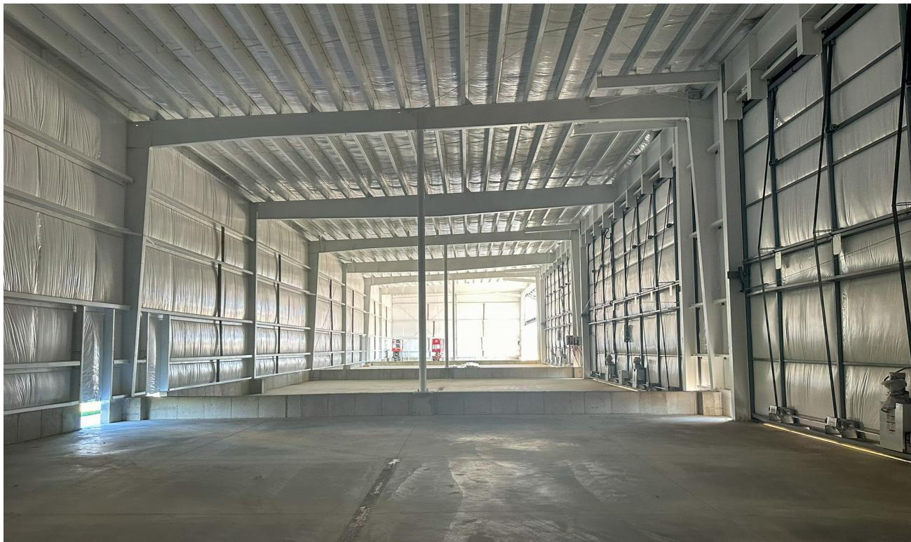
Each hangar allows tenants to store one or two aircraft and easily accommodates future insulation and heating, should individual hangar tenants choose to heat their units
