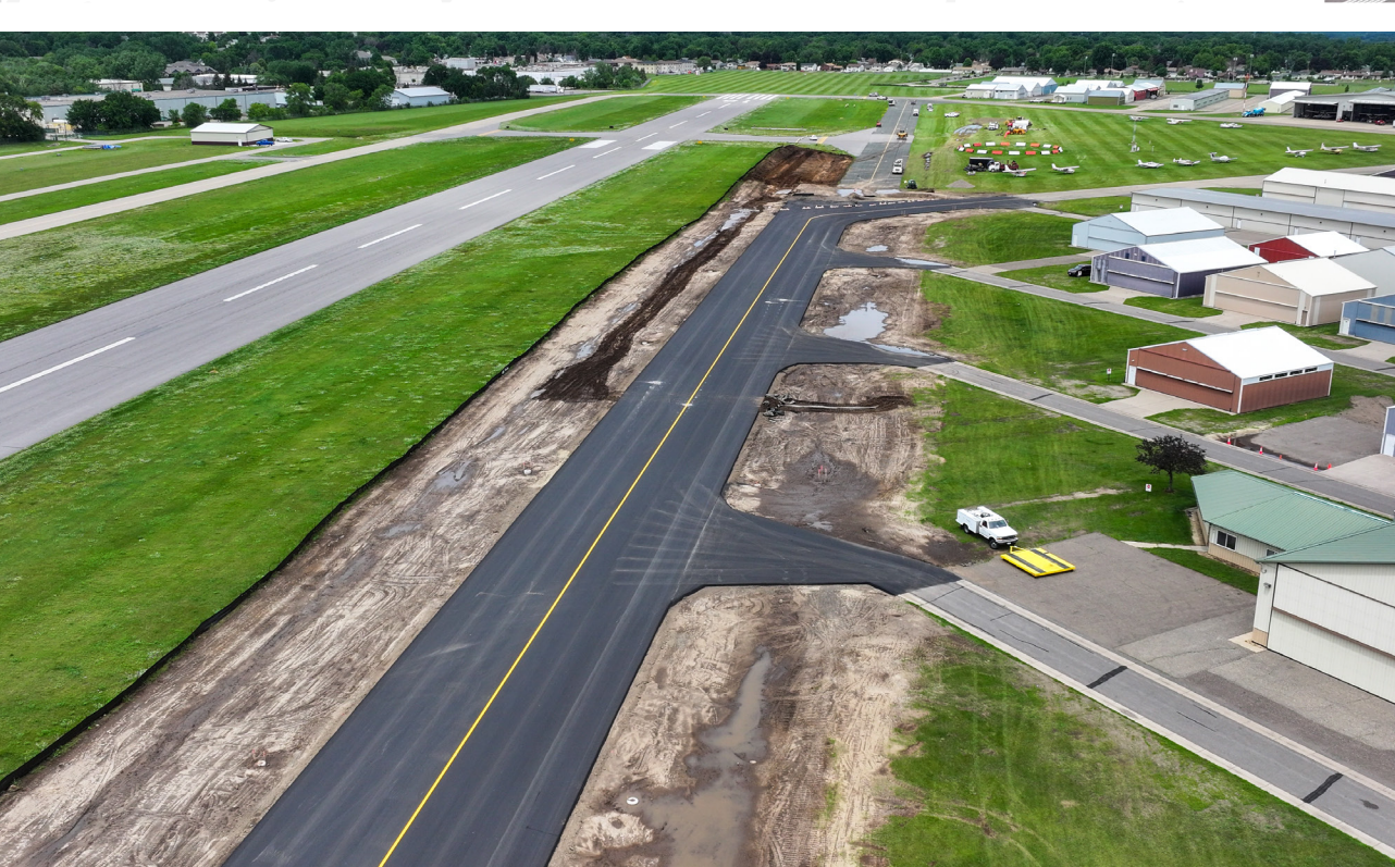
A recent Triggering Event Master Plan (TEMP) study recommended a shift in the existing Taxiway A alignment.
