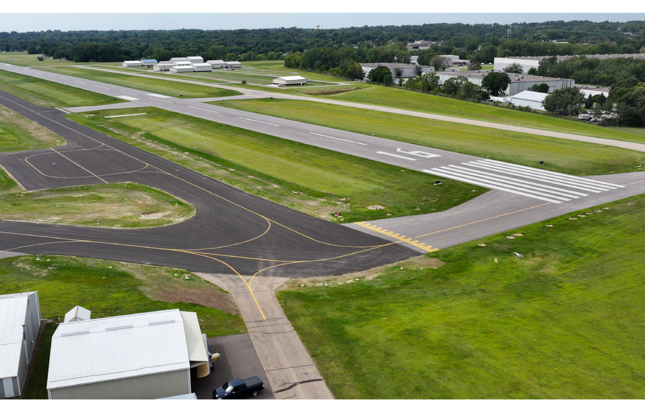
The newly reconstructed Taxiway A utilized reclaimed bituminous pavement and aggregate base from the existing Taxiway A.
