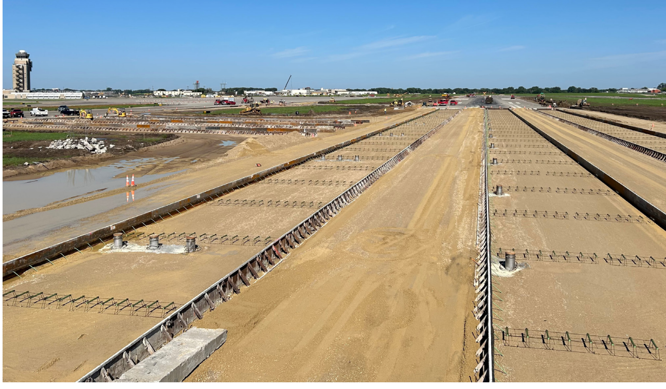
Closing Runway 12L-30R doesn't occur often, so the design team completed as many maintenance projects as possible during the closure
