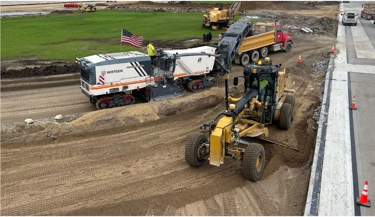
The project adopted an aggressive schedule to minimize airport impacts during certain weather conditions, requiring the contractors to work long hours and weekends
