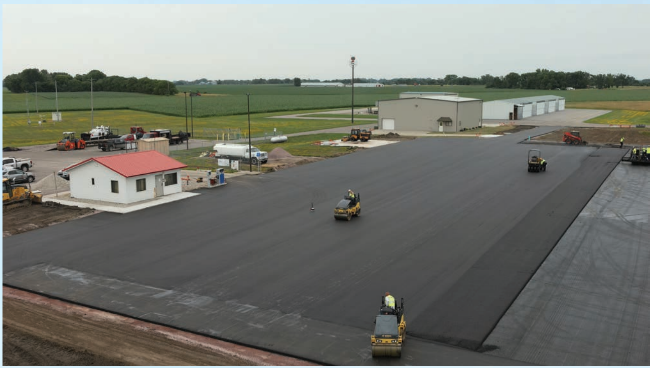
TKDA designed several different pavement sections to utilize as many existing salvageable on-site paving and base materials as possible, which helped reduce project costs.
