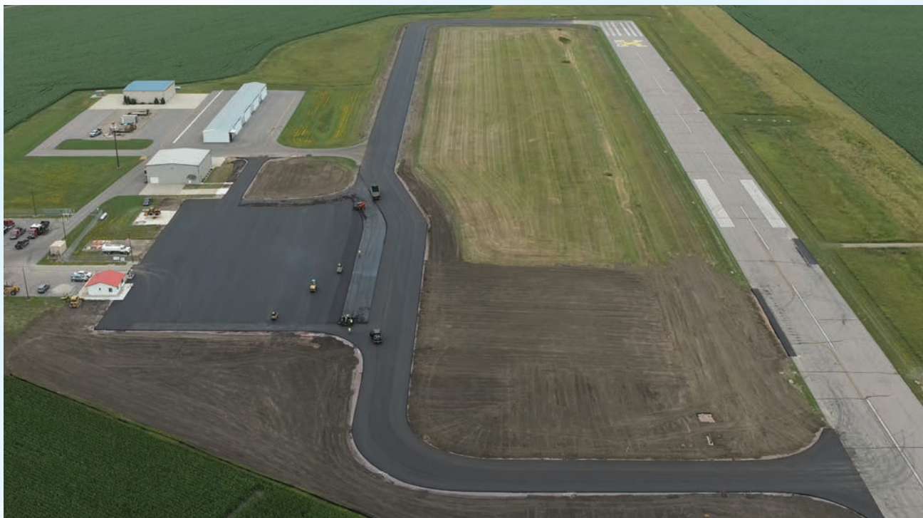
Connector Taxiway A was relocated to eliminate the direct connection to the runway, in order to reduce the likelihood of runway incursions, and come into compliance with current FAA design guidance.
