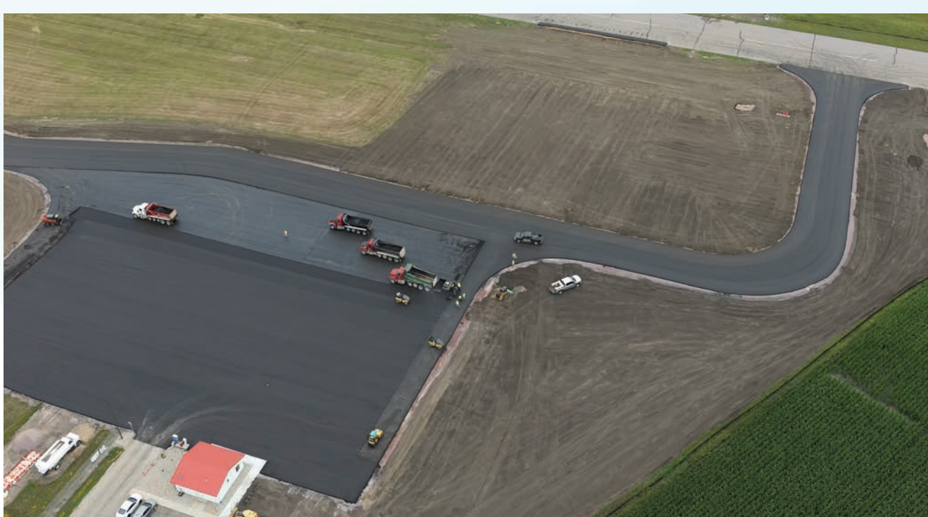
The project included slightly expanding the apron to provide better tie-down areas, ensuring parked aircraft would not impede access to the fueling area or taxiing aircraft.
