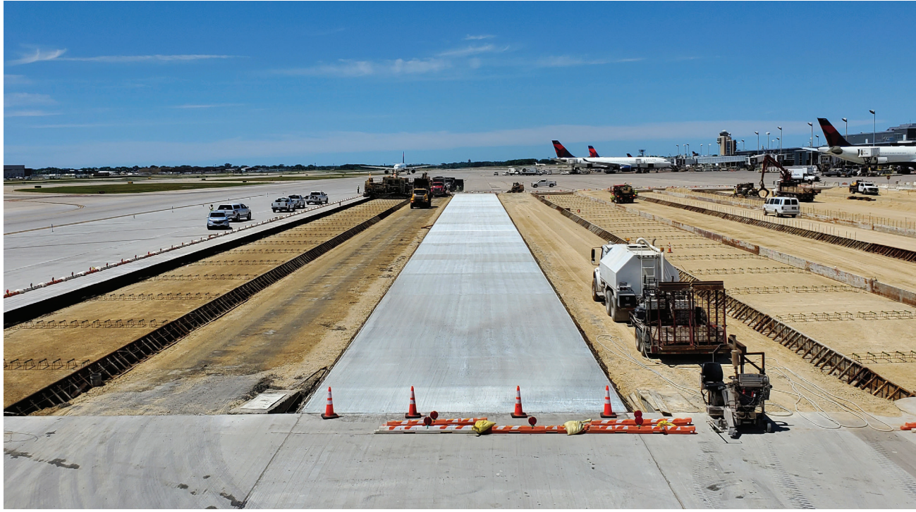
A concrete pavement section was assessed and designed for the taxiway and aircraft apron areas to support new and future aircraft
