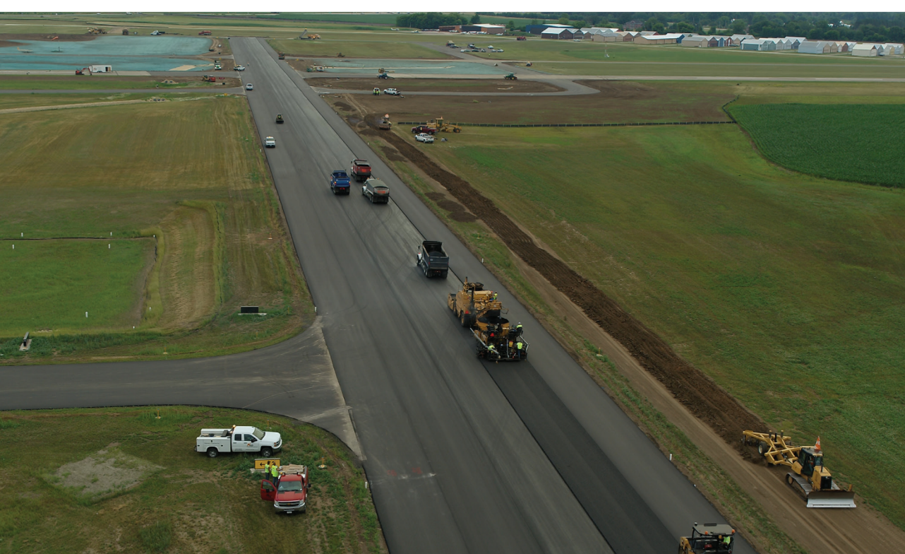
Tight construction schedules to minimize airport impacts meant multiple simultaneous operations: paving, electrical, edge grading, and seeding.
