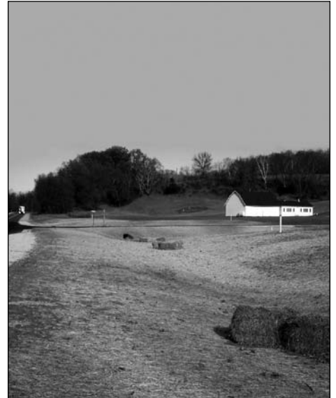
Fig. 2. Ditches direct water away from the roadway base. Hay bales in the ditch reduce flow velocity.
